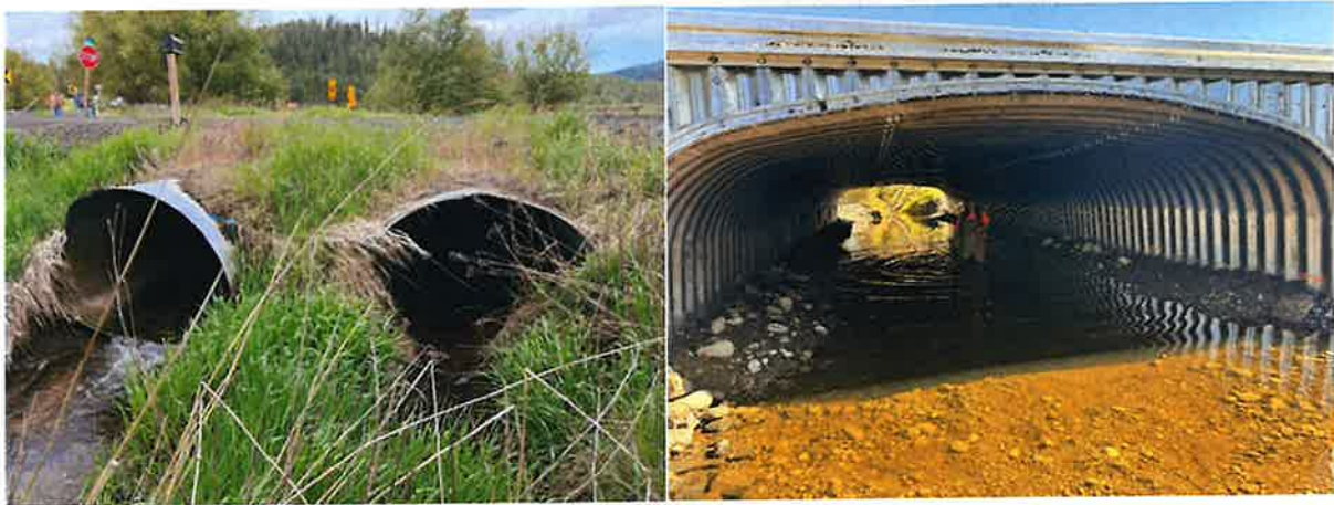
West Fork Lake Creek culverts before (left panel) and after (right panel) construction.
