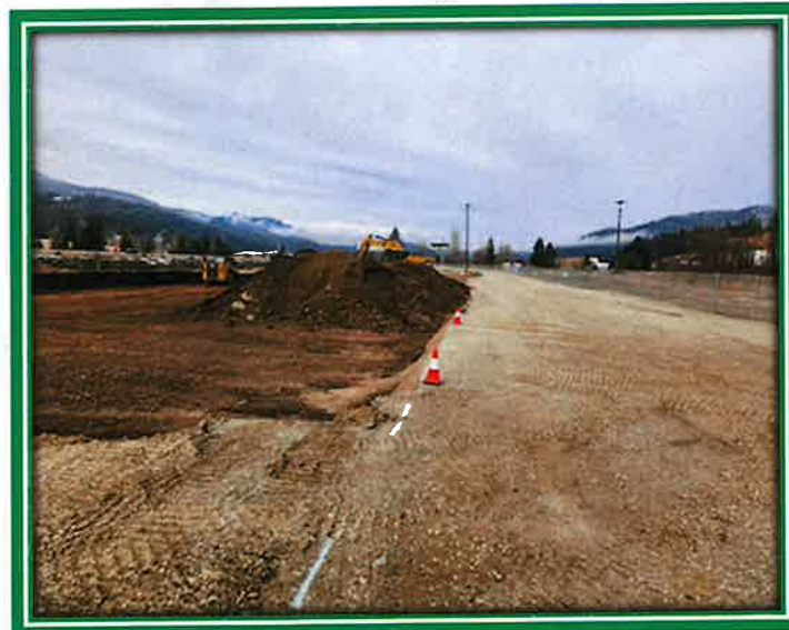
Facing west showing excavation of top foot of contaminated soil along south edge of Theater Bridge Road. Photo courtesy of Idaho Department of Environmental Quality.
