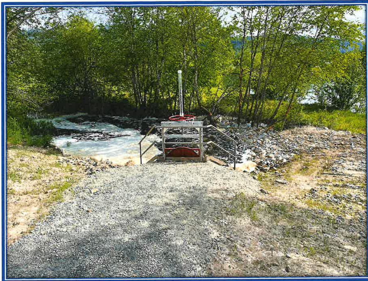
Pump Discharge Structure on the North Side of Trail Gray's Meadows Project
