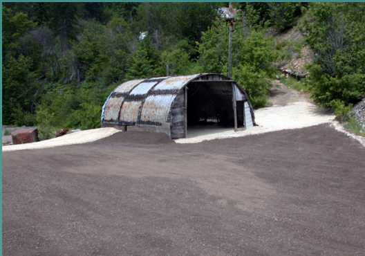
Excavation of contaminated materials and backfill of clean materials completed. Sod or grass seed will be placed next.
