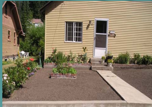
With backfill of clean soil complete, sod or grass seed will come next.
